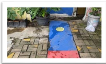
Figure 1. Condition of the work area floor made of paving blocks
